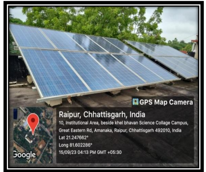
Roof Solar panel
